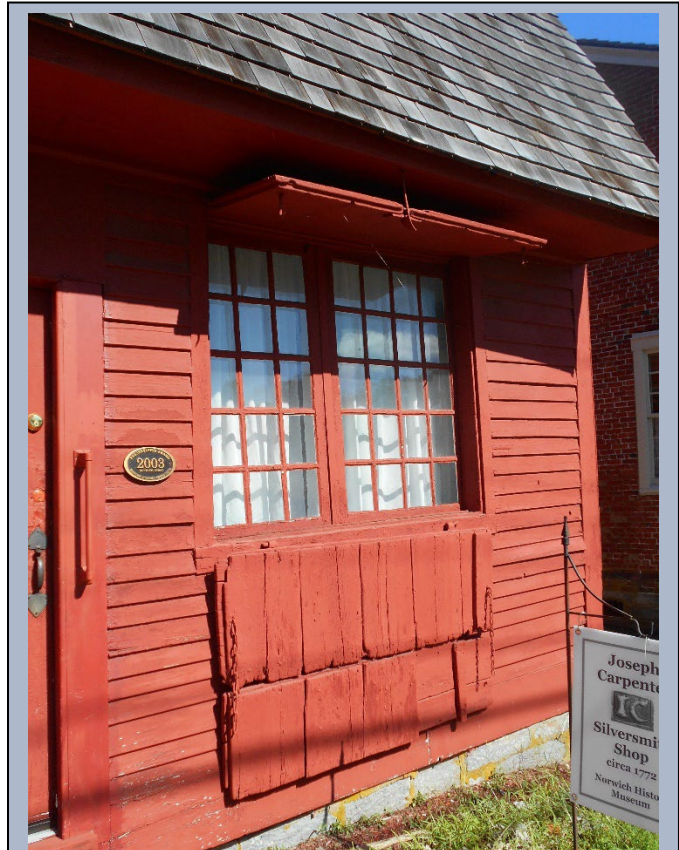
The exceptional design of the shutters on the Joseph Carpenter Silversmith Shop are an example of character defining features on this building.
